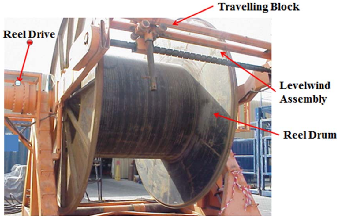
Figure 3-4: Coiled Tubing Reel unit
